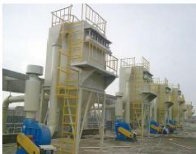
Dust collector installation site
